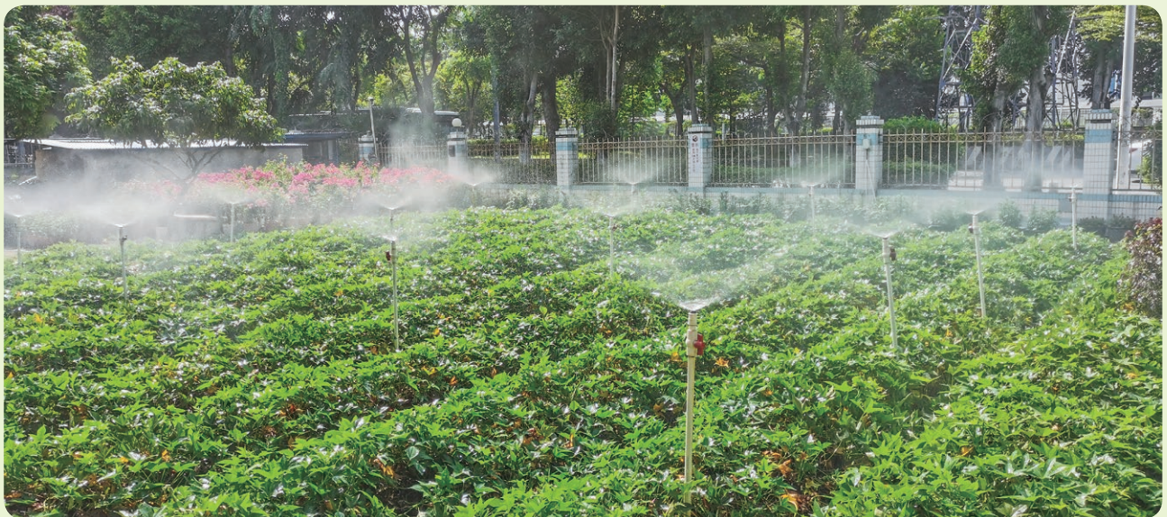
Rainwater Harvesting System at VTech Factory
